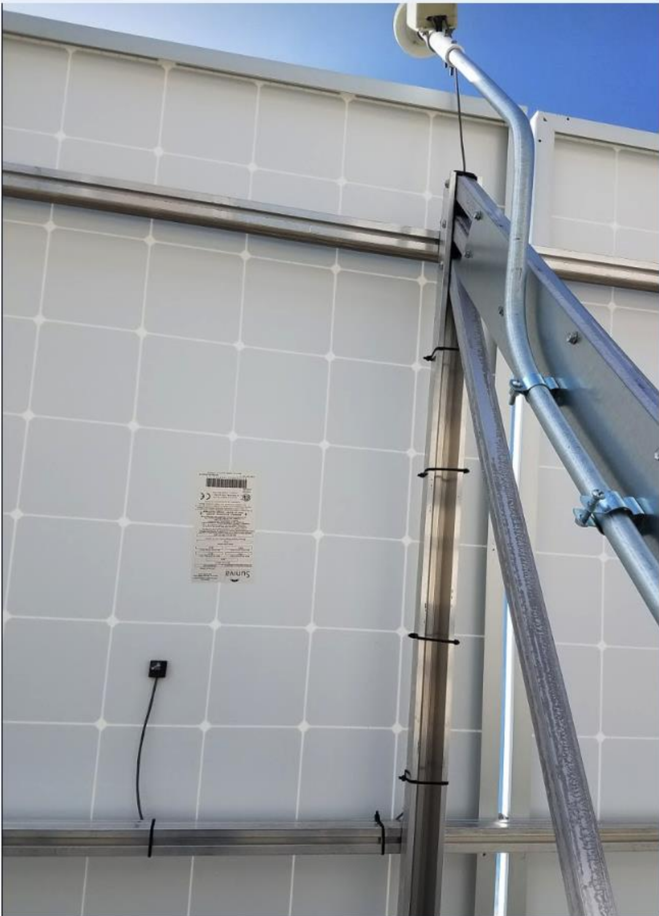
PV Solar System Efficiency Summer 2017:
